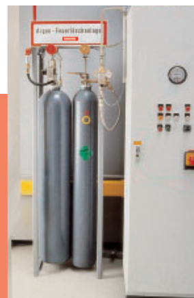
Extinguishant cylinders for gun- and filter protection
